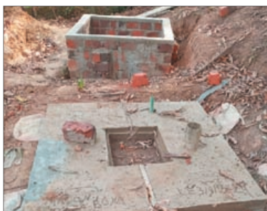
Casing of the well and the lid
